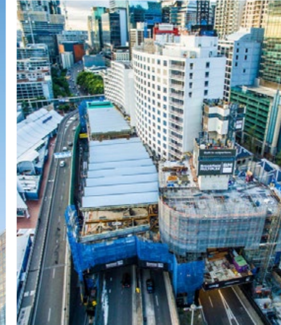
Hyatt Regency Hotel \ Situated over the Western Distributor motorway, the success of this project relied on close collaboration to ensure constructibility of design within a highly constrained environment
